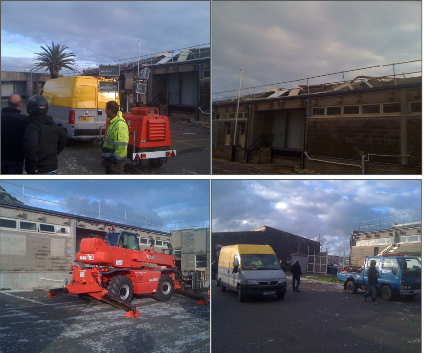
(above) The SteelMac team arrive and begin to repair the damage caused by strong winds
