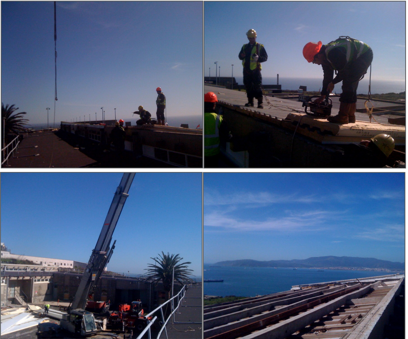
(above) Better weather helps the SteelMac team deal with the repairs quickly
