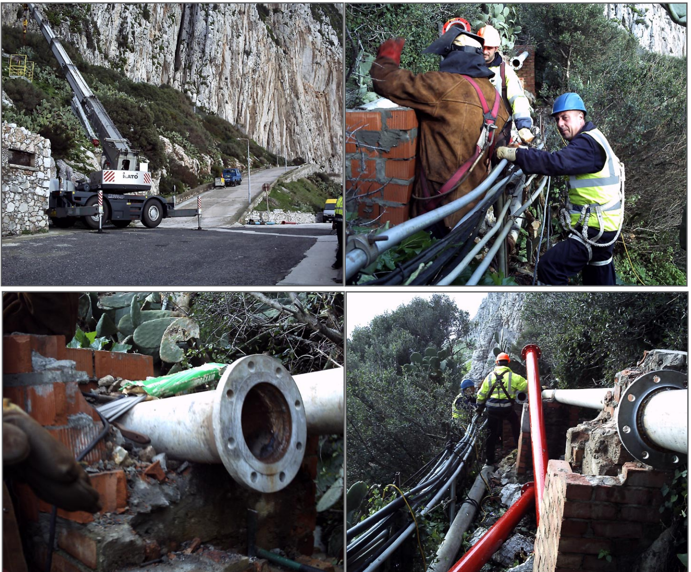
(above) Under the the supervision of J C Robba, the SteelMac crew complete vital repairs to the Fire Main Line
