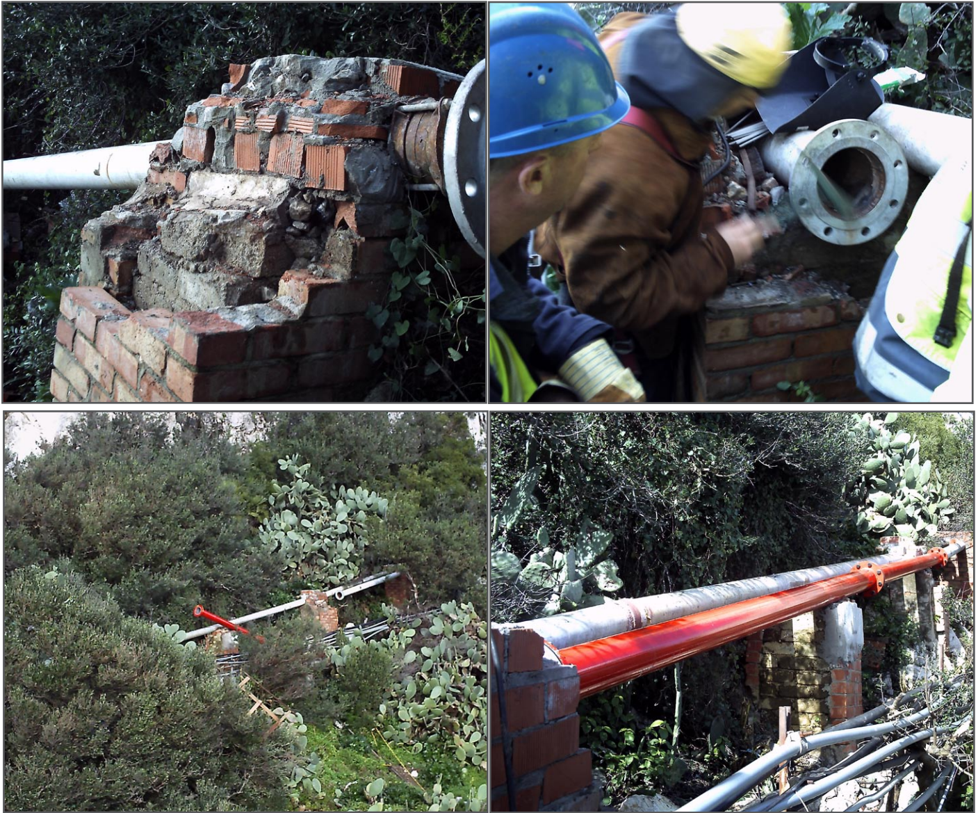
(above) The new pipework is installed and the supports are repaired to allow for greater stability
